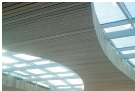
The challenging roof design at Highcross Mall featured inward- and upward-curving skylight areas.
